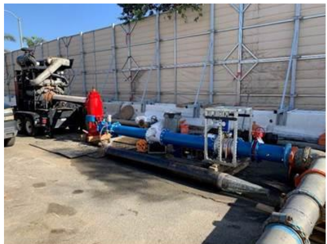
Injection Well Testing, Sound Walls Visible Behind
