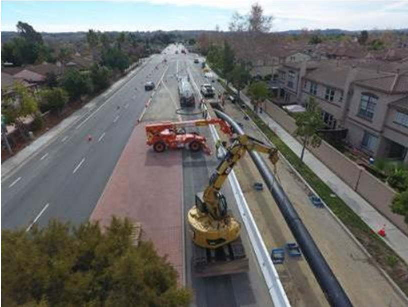
Recycled water external casing for river crossing
