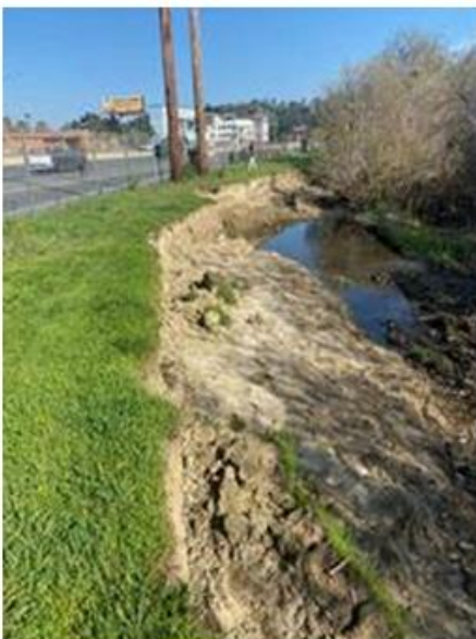
Figure 1 - Before the Repairs (January, 2020)
