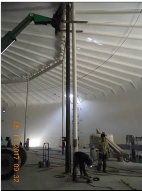
One of the columns is being replaced and will be coated after welding.
