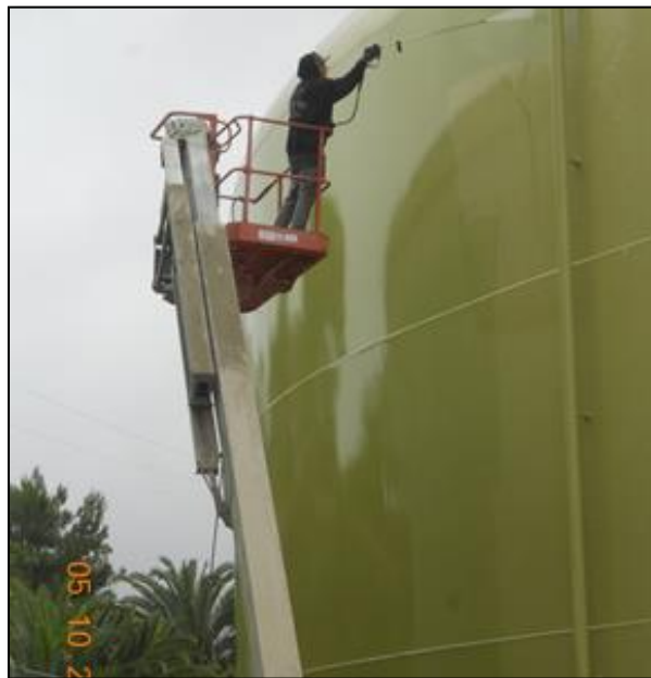
Tank is power washed in preparation for spot sand blasting and final coating.
